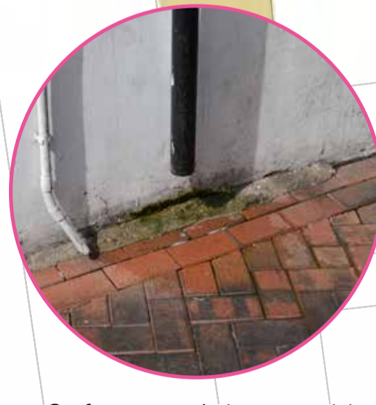
Surface water drainage provision is variable throughout street Inadequate drainage gullies and down pipes discharging onto road surface with no channelling or low spot - some in areas of café seating
