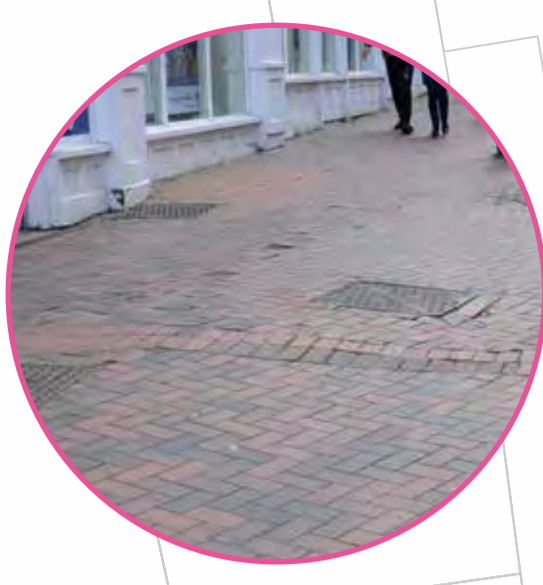
Clay pavers with uneven surface. Deformation suggestive of inadequate sub-base and/or water ingress
